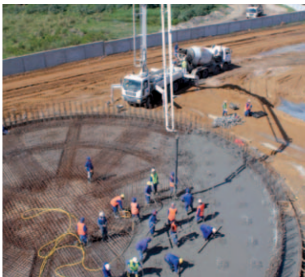
CMC Africa Austral's $36 million sewage system plant, opened in 2007, is benefiting 290,000 inhabitants of Beira
